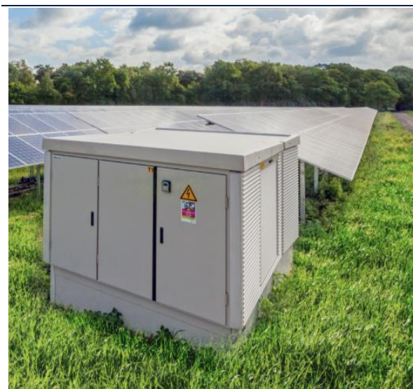
Fig. 47: Transformer substation in the Netherlands
